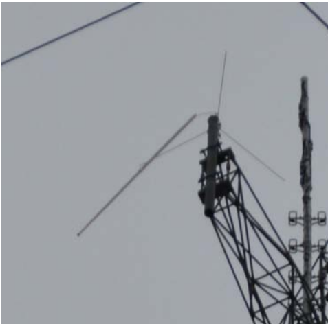
Tornado damaged remote repeater receiver antenna on the Diamond tower Story on page 3
