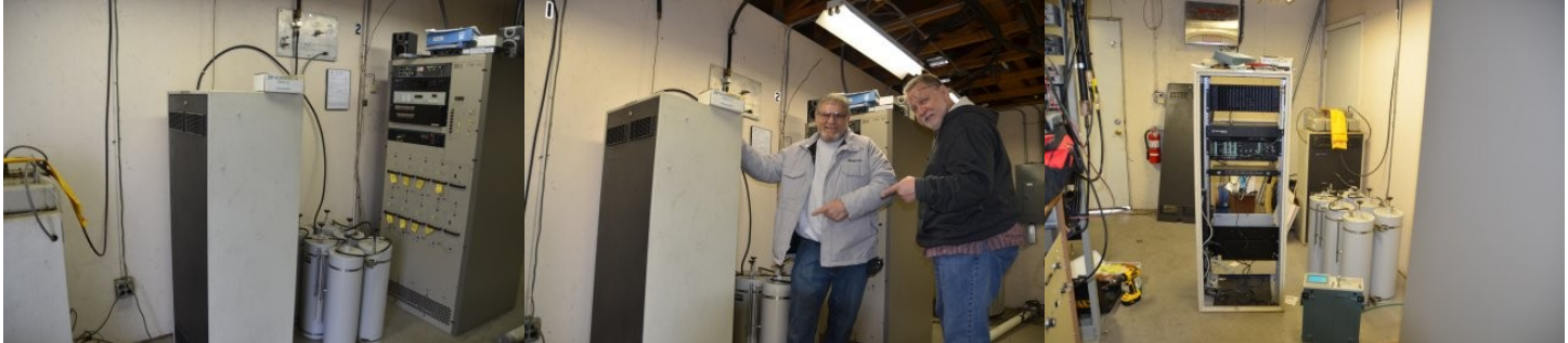
The 145.130 repeater and duplexers sitting in front of the WKCC broadcast transmitter
