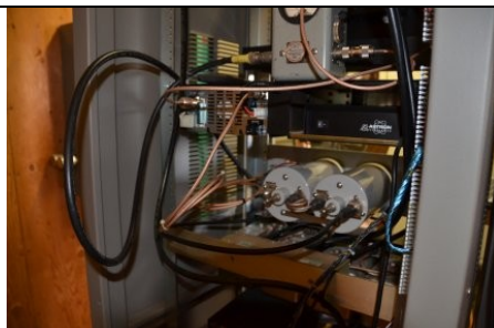
Inside the 440 Repeater. One of the 3 that received a new controller.
