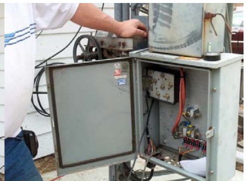
An inside view of the control box showing the tower wiring and a remote coax switch -N9RJM
