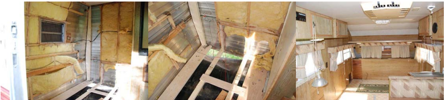
Rear inside view with bathroom area removed and water damage issues being addressed
