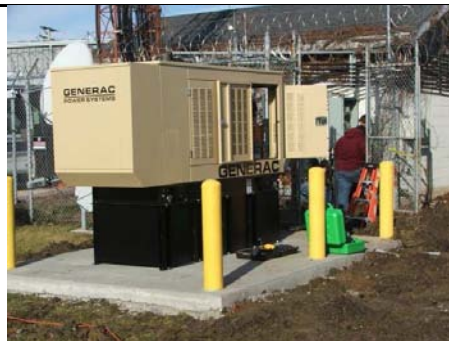
KARS 34/94 repeater will be on the air to relay emergency and weather messages even during power outages
