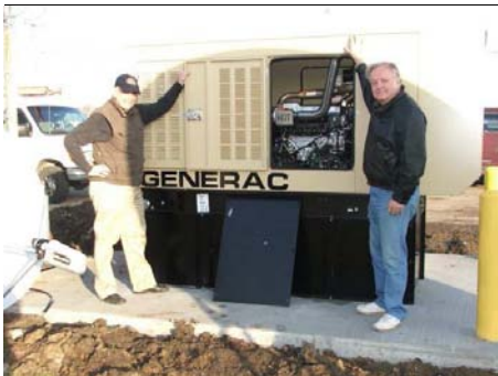
Howard AK9F and Don K9NR are pictured next to the new Generac 80,000 watt diesel generator.
