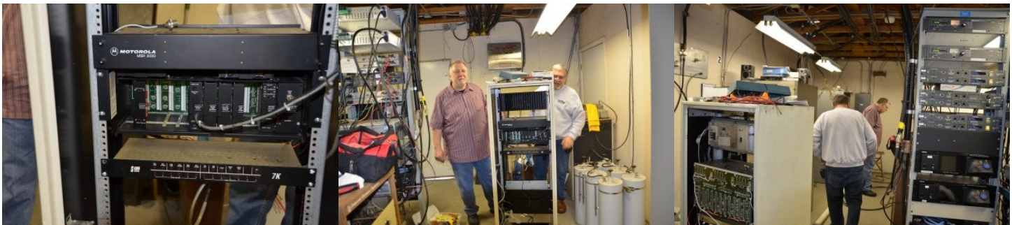
A view of the Motorola MSR2000 repeater and SCom controller... the 100% duty cycle power supply and 100 Watt final amplifier are not visible.
